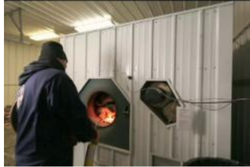
PICTURE 5: GARN BIOMASS BOILER (KOYUKUK, AK)
